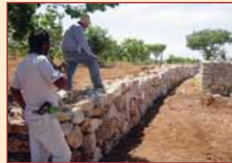
Restoring agricultural land through the construction of stone terraces in Beit Jala
