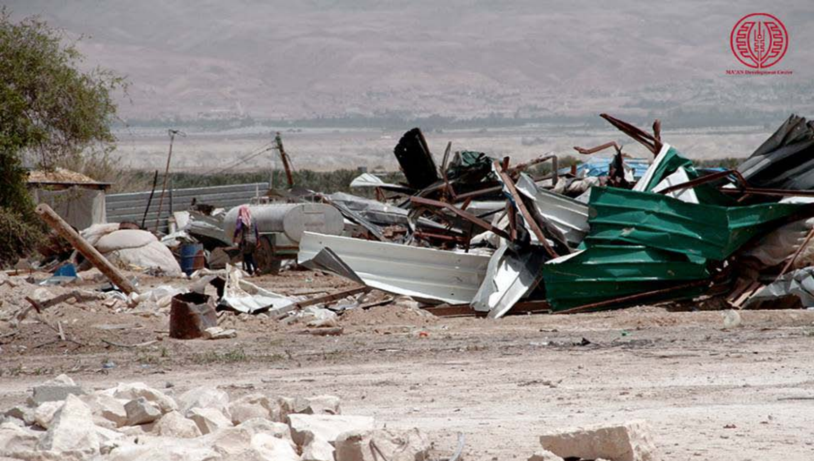
Residential structures in Jiftlik, central Jordan Valley after they were demolished by the Israeli army
